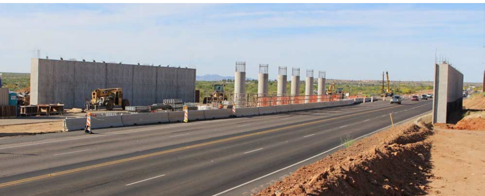
A boring construction site? No, it's Pima County's first wildlife bridge taking shape on Oracle Road. Thank you for helping the Sonoran Desert's first wildlife bridge become a reality! Photo by Terry Minks
